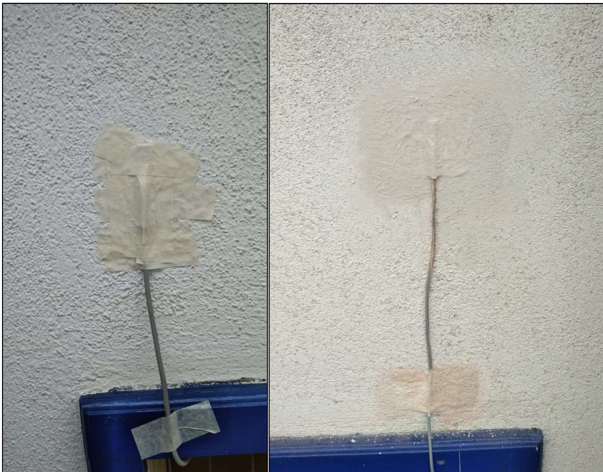
Figure 14-15 External surface temperature sensors before and after applying the lime paint protection layer
